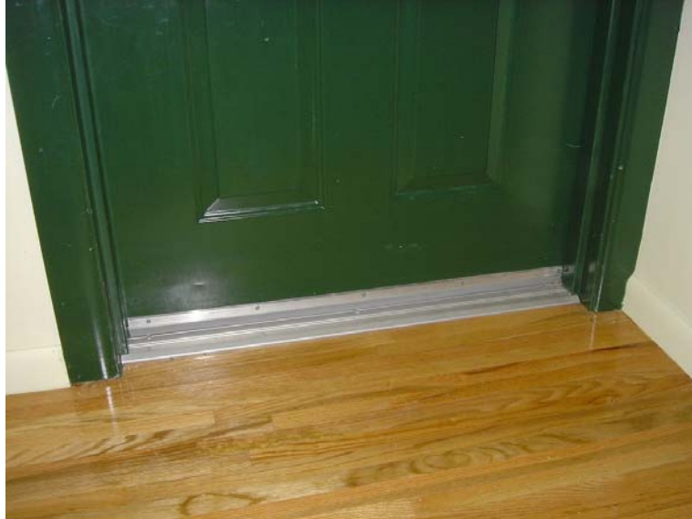
Figure 5: Weather-stripped corridor doors - Ventilation air is prohibited from being introduced into multifamily units from corridors; multifamily unit to corridor doors are typically weather-stripped
