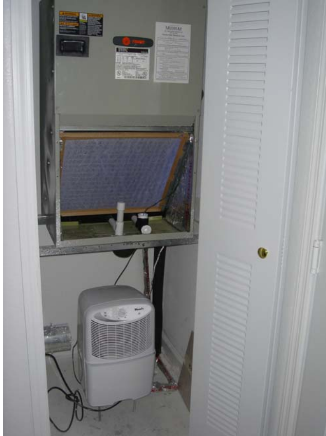
Figure 20: Dehumidifier – Located in return closet
