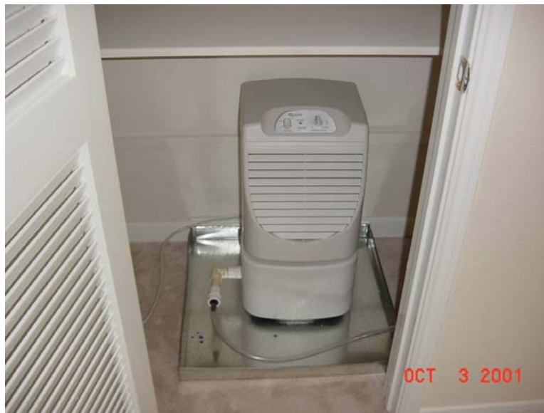
Figure 21: Dehumidifier – Located in closet with louvered door
