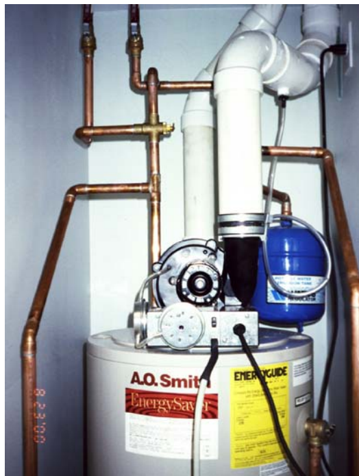
Figure 15: Gas water heater - Gas water heaters if used should be sealed combustion two-pipe systems vented directly to the exterior with combustion air ducted directly to the water heater
