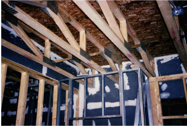
Figure 3: Common wall construction – Common walls are required to meet fire and smoke assembly requirements
