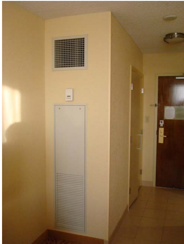
Figure 13: Individual unit space conditioning – Each unit has its own air distribution system
