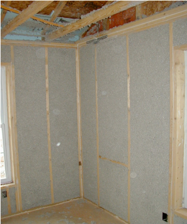
Photograph 1: Increased Thermal Resistance—Lots and lots of thermal insulation in the building enclosure. Spray applied cellulose with insulating sheathing in a wood frame wall.
