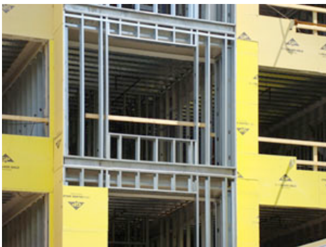
Photograph 6: No Hygric Buffer—Not a lot of moisture storage in hollow steel stud walls sheathed with gypsum.
