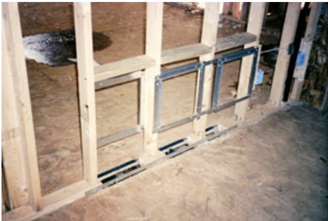
Photograph 7: Sucking on a Wall—Stud cavity return system couples interstitial cavities directly to the HVAC system.
