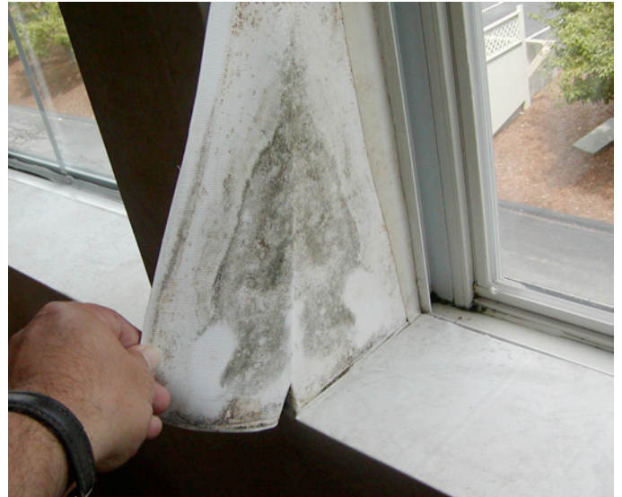
Photograph 3: Vinyl Wallcovering—Bad, very bad, very bad indeed.
