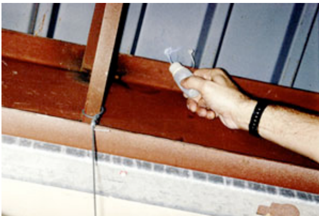
Photograph 9: Sucking on a Wall Part Deux—Commercial return plenum draws air out of exterior walls into the return side of the HVAC system and then subsequently connects to the breathing zone of the occupied space.
