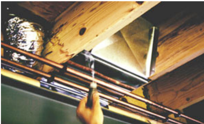
Photograph 8: Sucking on a Floor—Panned floor joist return system couples floor framing directly to the HVAC system.
