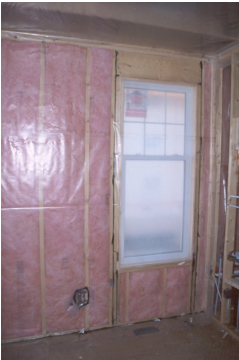
Photograph 2: Impermeable Interior Lining—Polyethylene vapor barrier on the interior of a wood frame wall causing mischief.
