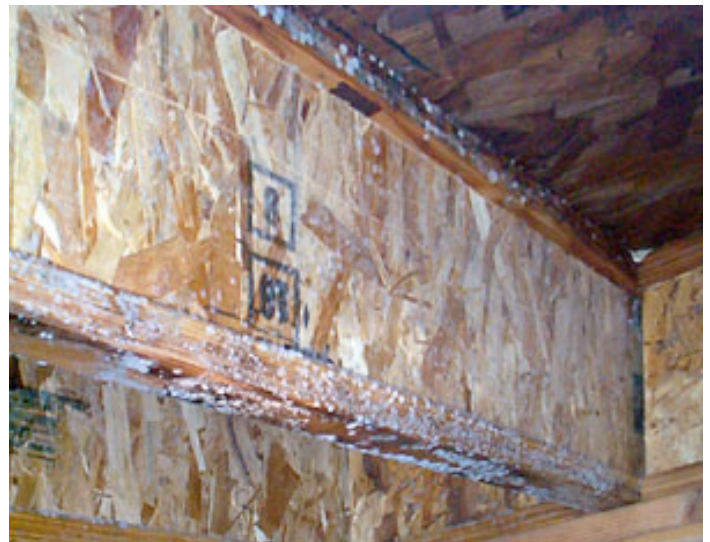
Photograph 4: Mold Sensitive Materials—Engineered wood materials manufactured from OSB and composite wood layers. Mold food par excellence.
