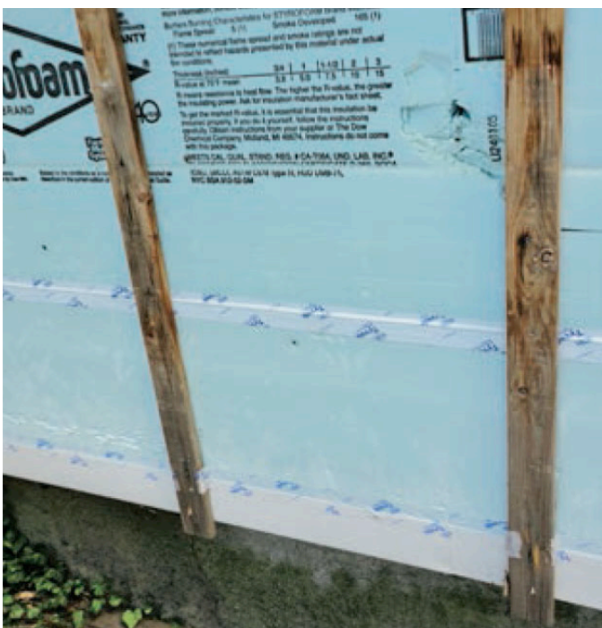
Photograph 8 (left): Sheathing Tape Works —Look at how good this looks after 15 years. That is not new tape; that is 15-year old tape. Awesome. Note the aluminum C-section at the bottom of the blue XPS capping the bottom protecting it from critters. Note how good the untreated wood furring looks.
