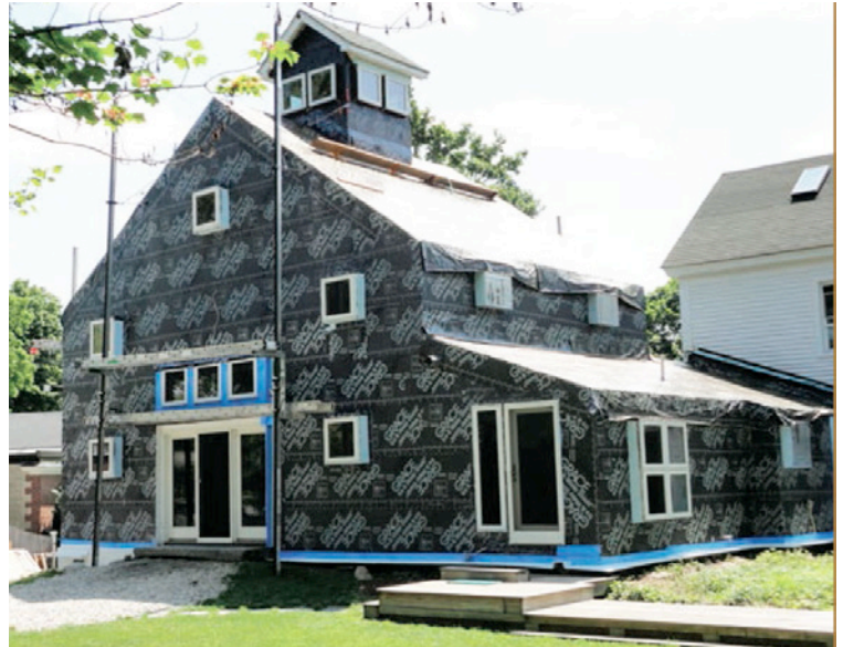
Photograph 12: Control Layers —An even more beautiful sight: a fully adhered membrane acting as a water control layer, air control layer and a vapor control layer. Reverse laps are taped with sheathing tape. No more poly for me.
