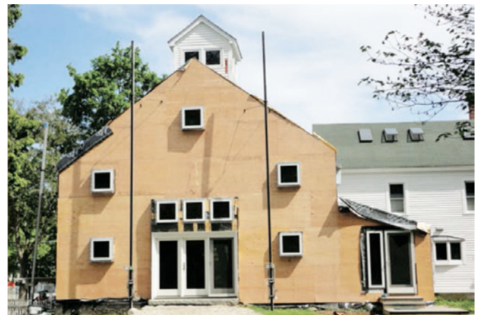
Photograph 11: Shear Control —A beautiful sight: plywood structural sheathing wrapping the walls and roof of a hundred-year board-sheathed timber frame. Bring on the nor'easters.
