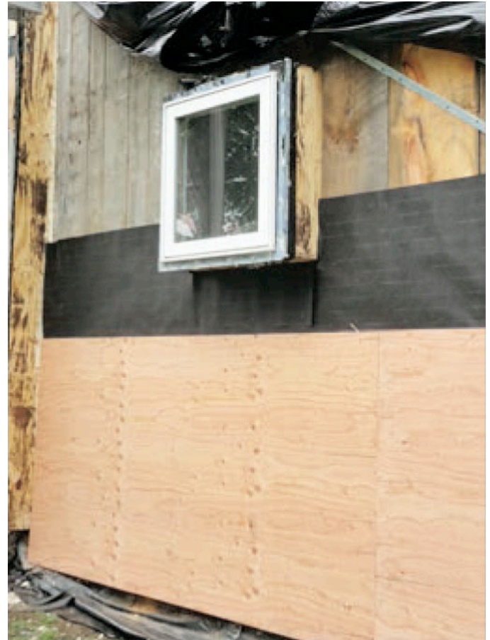
Photograph 10: New Wall —Note the “new” tar paper on the old barn boards under the new plywood structural sheathing.
