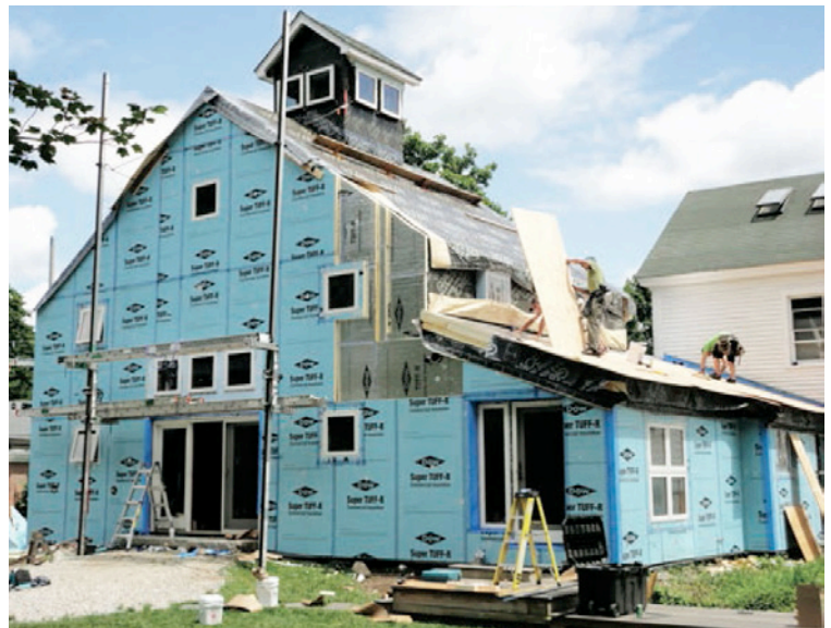
Photograph 13: Thermal Control Layer —Note the four layers of rigid insulation on the walls and the five layers of rigid insulation on the roof. You had better believe that each layer was offset horizontally and vertically and that each layer was sealed. I watched every sheet go in this time. None of this “faith-based” stuff anymore.
