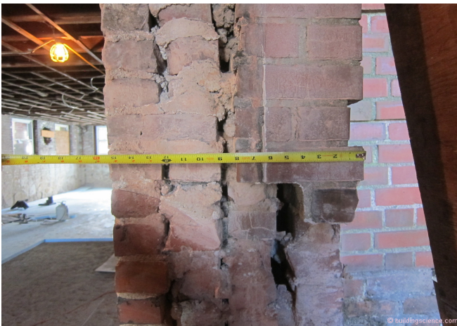
Photograph 3 – Brick Wall Section: Solid mass walls are not typically solid. Let me repeat...solid mass walls are not typically solid.
