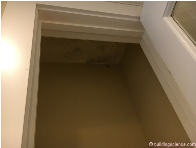
Photograph 6: Mold in Closet - We now get mold inside the home at closet ceilings. When we couple the colder closets with higher levels of ventilation air you need to add supplemental dehumidification or you have to provide closet ventilation or both. Sure would be nice if sales and marketing would let us go back to louvered closet doors.
