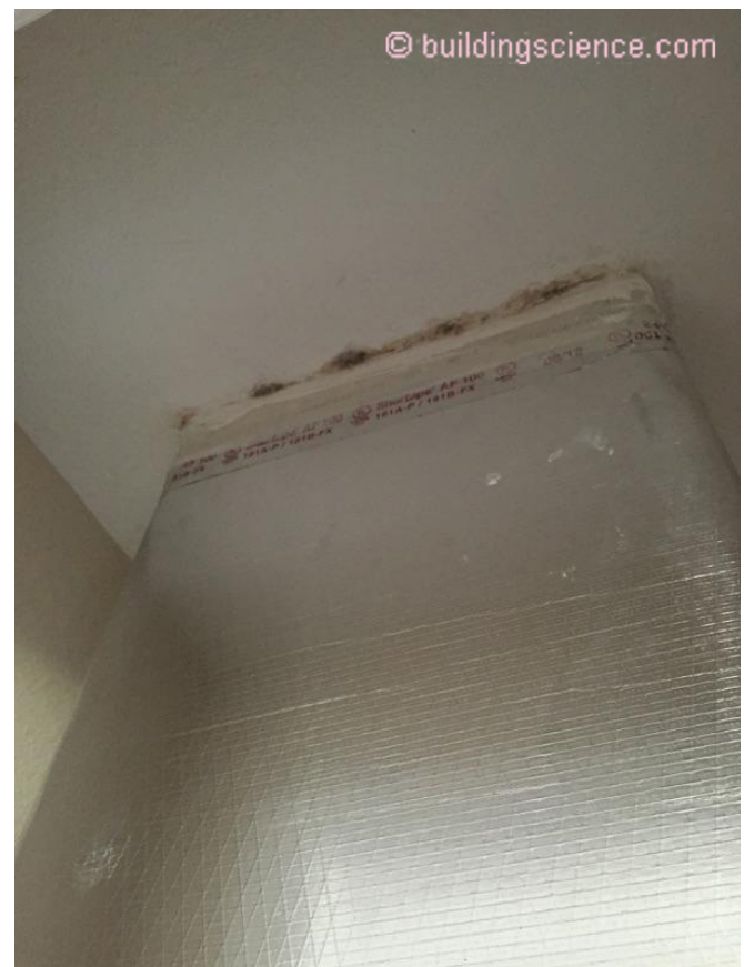
Photograph 7: Mold on Supply Plenum in Mechanical Closet - Don't forget to increase the insulation levels around the supply plenum where it penetrates the mechanical room ceiling.
