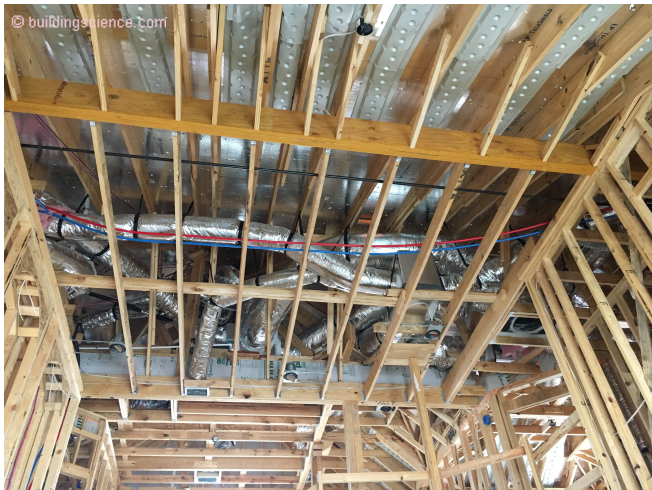
Photograph 4: Radiant Barrier – The “shiny” aluminum foil adhered to the underside of the roof sheathing is the radiant barrier.
