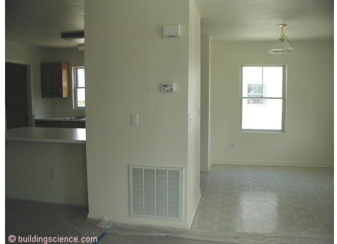
Photograph 1: "Filter Grille" - Remember the good old days when we had filters right at the single central return that we could easily change. We didn't have to go to the furnace or the air conditioner. The filter was right there.
