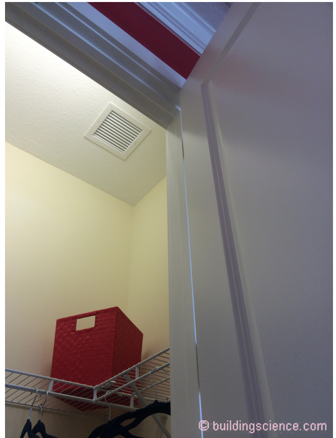
Photograph 8: Closet Ventilation - The best way to provide closet ventilation is to install a small return air duct in the closets. Guess what? Not “technically allowed” in the Florida Building Code or the International Residential Code. Be nice to your CBO.
