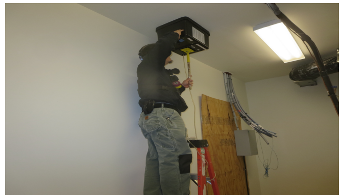
Figure 17: Exhaust fan flow meter
