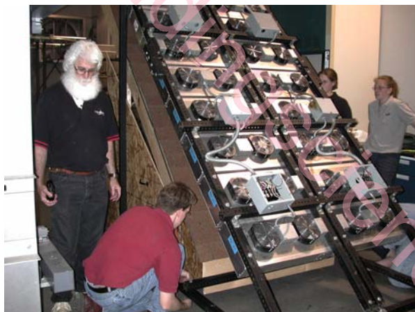
Figure 2b: Roof with solar array
