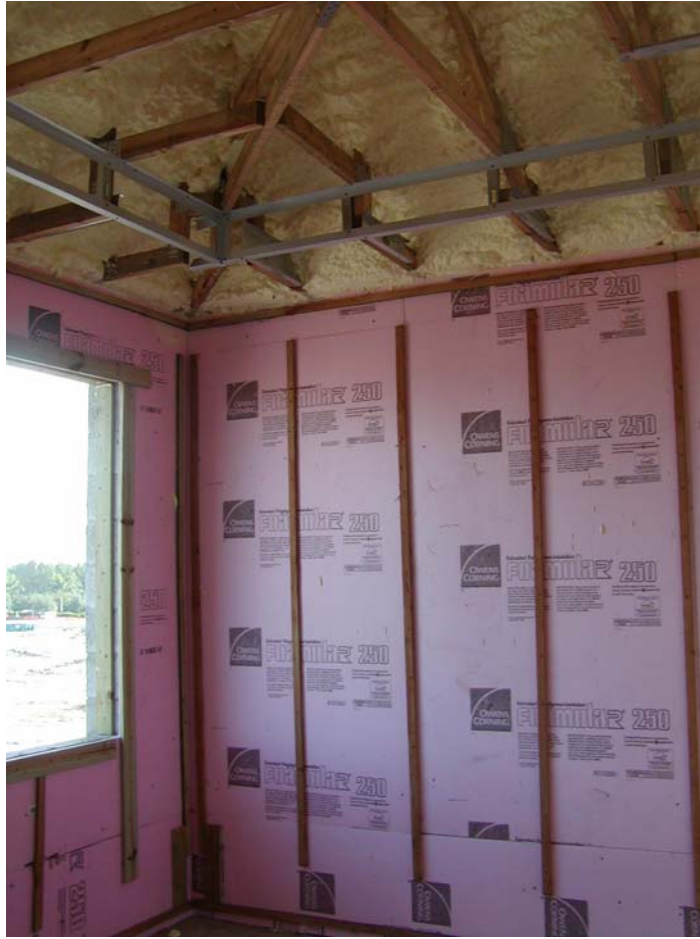
Photograph 7: Non-Water Sensitive Interior Insulation. “Note the unvented conditioned attic using vapor open spray foam – conditioned attic is preferred location for HVAC system.”
