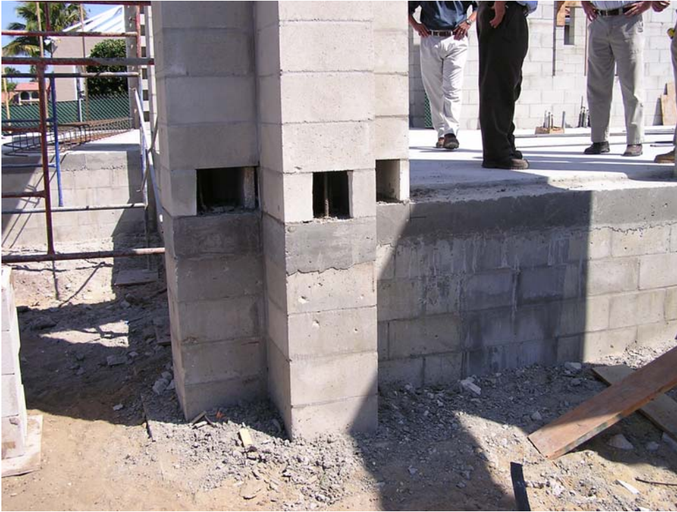
Photograph 3: New Home Under Construction – Ft. Myers, FL. "Note the elevated slab relative to the surrounding grade and the non-water sensitive structure (masonry wall)
