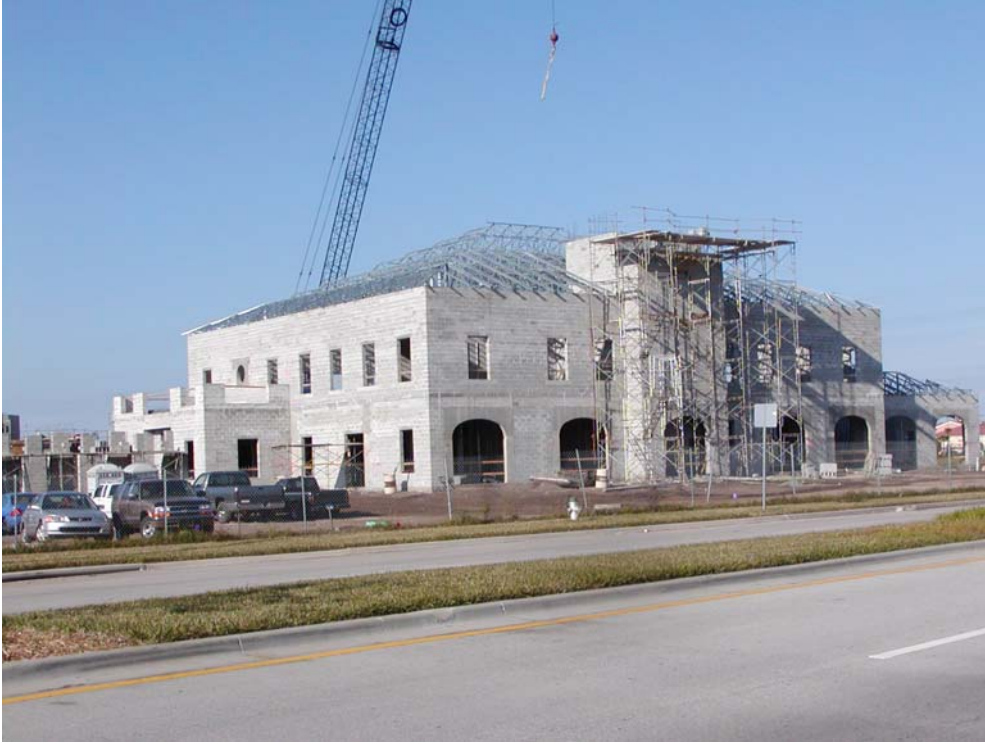
Photograph 4: Commercial Office Under Construction in Orlando, FL. "The basic structure is constructed from completely non-water sensitive materials – the building has 'good bones.'"
