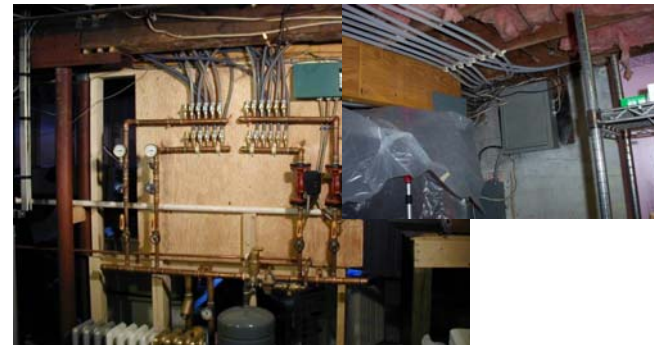
Manifold Distribution – home run to every radiator
