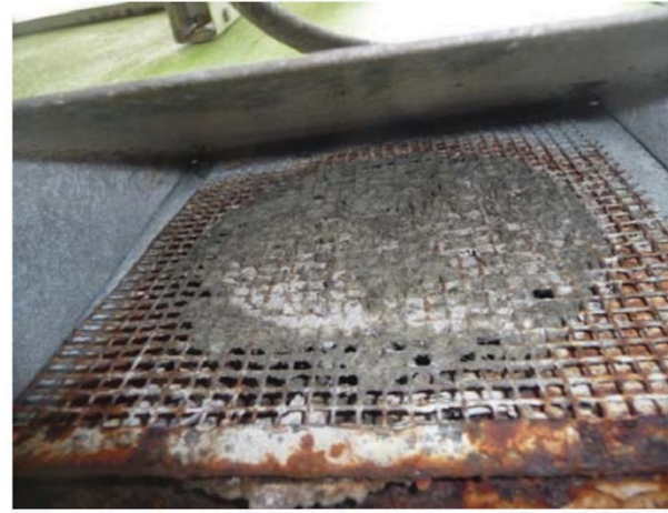
Dirty outdoor air intake.
